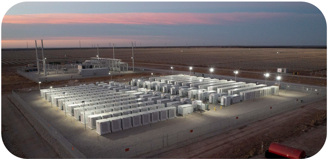
Figure 1. Example of a BESS Project
